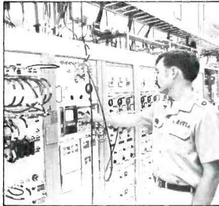
Chief Warrant Officer Stephen Dill makes an adjustment to a Spectrum Analyzer used to measure power. The East Coast Telecommunications Center is part of a worldwide satellite communications network.
